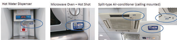
Figure 1 – Over 50,000 items have been labeled and tracked using QR tags. These tags are regularly updated to monitor the item’s health and functioning over time.
