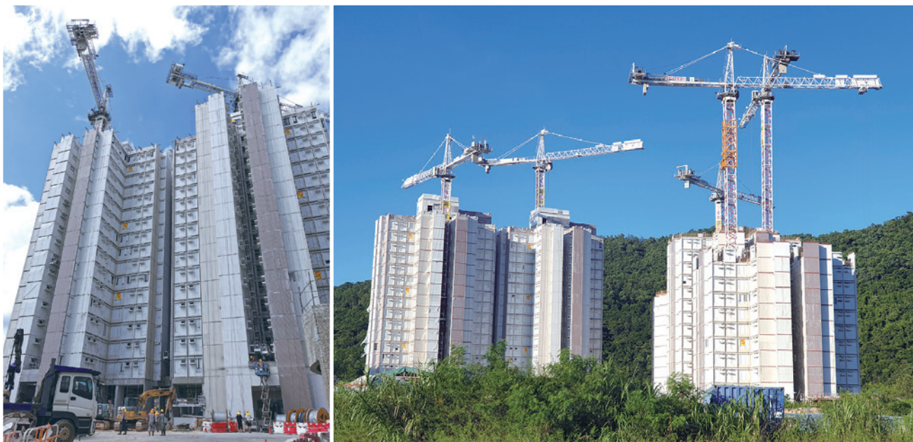
Hong Kong's first concrete MiC project — the Disciplined Services Quarters for the Fire Services Department in Pak Shing Kok, Tseung Kwan O. 香港首個混凝土 MiC 項目——將軍澳百勝角消防處紀律部隊宿舍。(Photos provided by Sr Charles Hung)
