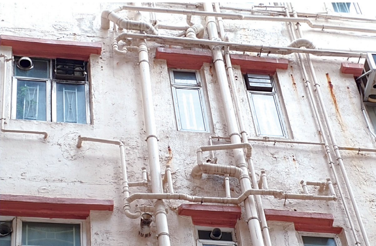
Typical crisscrossing branch pipes
