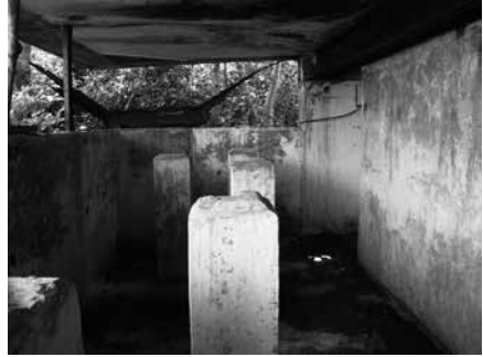
Figure 18: Pedestals for the plotting room on the ground floor of the observation post of D'Aguilar Battery
