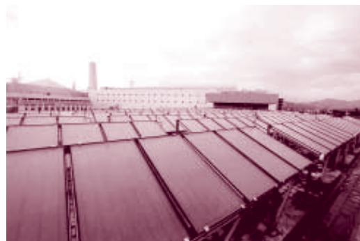
Solar hot water system on the roof top
