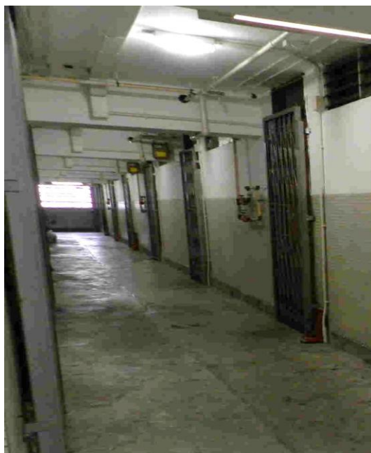
Picture 9a No Handrail in Corridor
