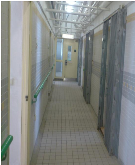
Picture 1 No Ventilation in Corridor
