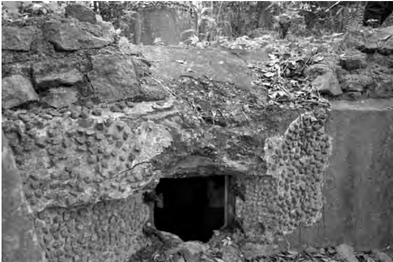
Fig. 5: Damaged eastern embrasure of PB 3
