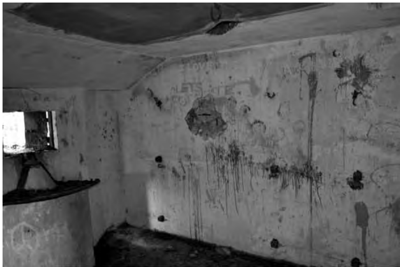
Fig. 7: Damaged wall behind the attacked embrasure (No similar damage of this size can be found in the pillbox)
