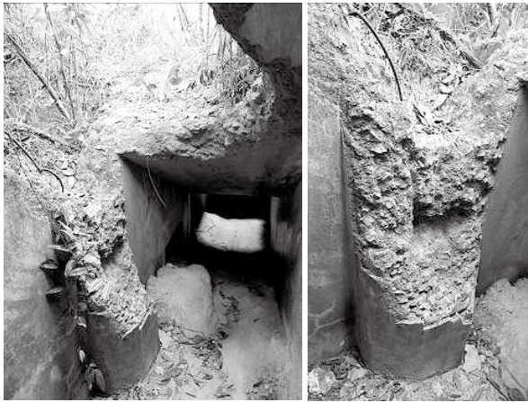
Figures 15A and 15B: The damaged bulge along the tunnel wall of Structure Y. Note the hole in the middle used to support the end of the steel rebar of the ceiling support beam.
