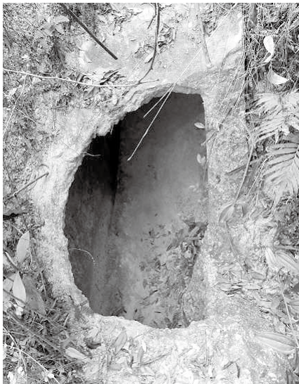
Figure 16: Damage to the tunnel roof.
