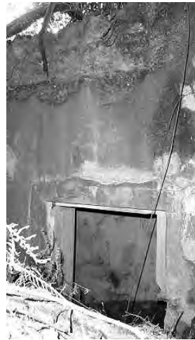
Figure 9: The entrance to the tunnel. Note: Note the damaged part on top of the wall indicating where a steel rebar inside the wall was removed.
