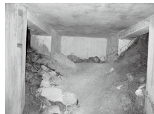
Figure 14: A short extension of the tunnel built to separate the two shelters and used as an entrance.
