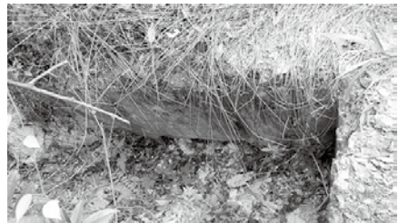
Figure 17: The shelter is almost completely filled by mud.
