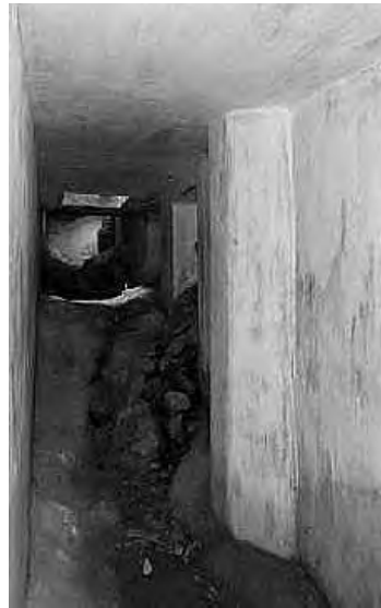
Figure 5: Bulge and opening along the tunnel wall in Shaftesbury Avenue. Note: The tunnel to Oxford Street is on the right side below the air vent opening.
