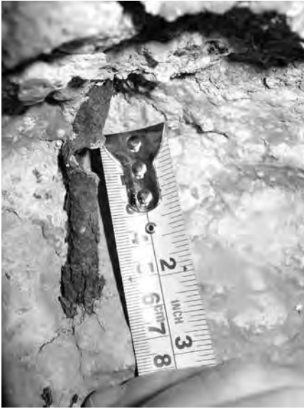
Fig 4: The almost severed reinforcement bar in the interior hit mark area. Note dimension c.6.5mm – the same as Japanese Model 96 LMG and Model 38 Rifle.
