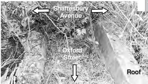
Figure 12: Looking from top of Oxford Street show the left and right side of the roofless structure. The top line of original roof is still visible.
