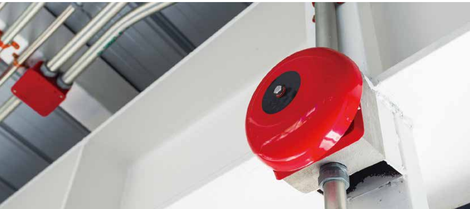
Older industrial buildings in Hong Kong that were completed before 1973 are not, at this moment, legally required to be fitted with sprinklers. (Photo: Thinkstock)
