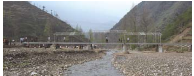
Last shot of the bridge from the upstream side just before the team left the field for home
