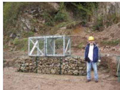
First steel framed gabion was completed on other gabions with stones to form the support for the bridge beams and decks
