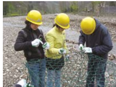
Student volunteers sewing the wire-mesh gabions to be filled with rocks for supporting the bridge beams and decks
