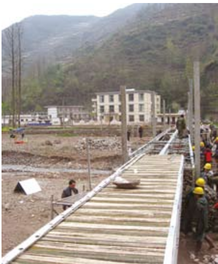
First section of the bridge decks was completed early on the third day
