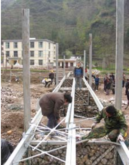
Twisted channels in the far end as compared with those squared and braced with the aid of hydraulic jacks and clamps
