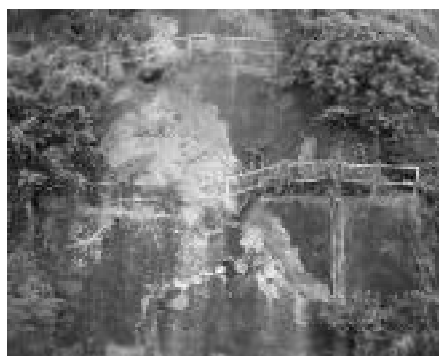
Plate 1: Cracks on failed slope
